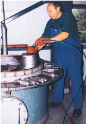
Manual cleaning of a vertical heat exchanger with flexible hose and bell-type splash guard.
